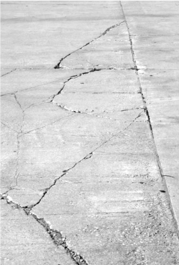
▲ Multiple slab cracks, spalling and shattered slabs.
