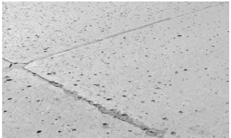
► Extensive pop-outs of large aggregate from surface.
