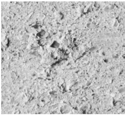
▲ Slight scaling. Minor loss of surface mortar.
