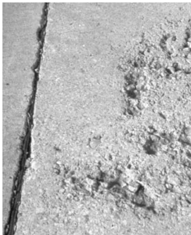
▲ Severe scaling. Joint and sealant in fair condition.
