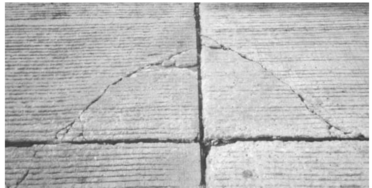
Corner cracking with slight spalling.
