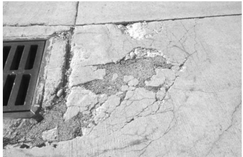
▼ Inlet with severe cracking and spalling. Full depth slab repair required.
