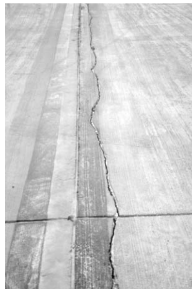
◀ Crack parallel to joint. Open 1/4". No spalling.
