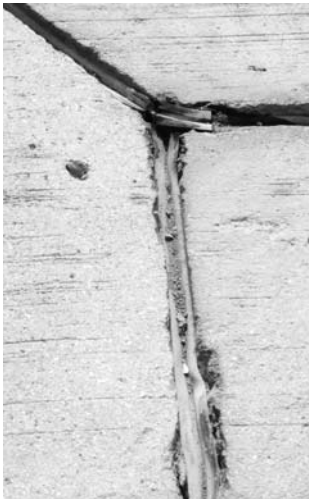
▲ Joint sealant in poor condition. Loss of bond to edge allows water into pavement.
