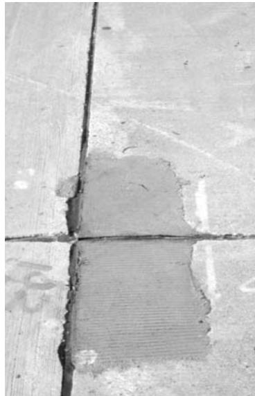
▶ Partial depth concrete patch to repair corner cracks. Good condition.
