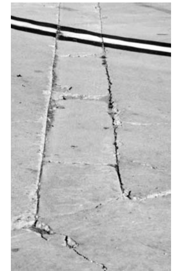
▲ Concrete patch in poor condition.
