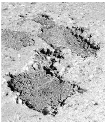
◀ Small surface spall that has been patched.
