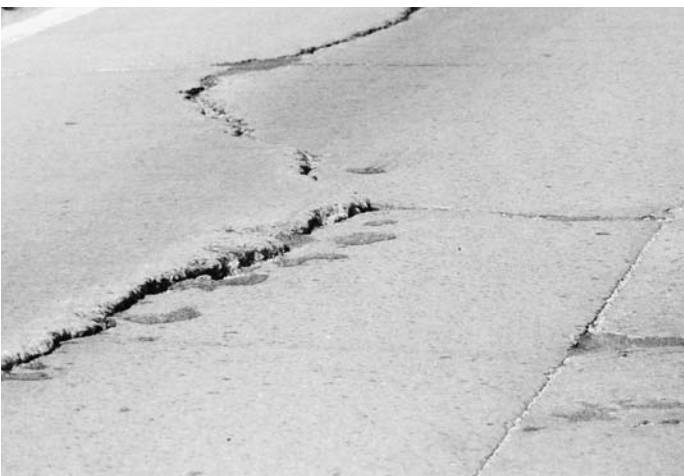
◀ Faulting and spalling of a meander crack.
